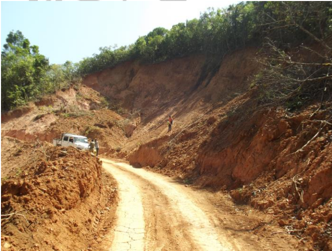
(g) Earth slide occurred on moderate to high slope which have affected the local road to north-eastern Niduvatu village
